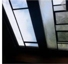
BEL Replace fogged window panes
